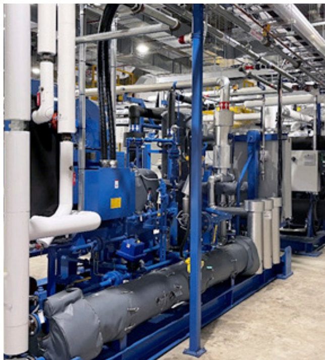
The Copeland CO 2 heat pump in operation at the Hydro Quebec Energy Technologies Laboratory in Shawinigan, Quebec produced 99.6 percent less Greenhouse Gas (GHG) emissions in testing.
